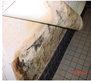
Leaks plastic laminate lack of caulk
