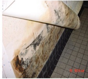
Leaks plastic laminate lack of caulk
